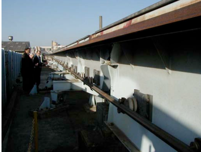
Figure 3-6. Side of HSST Guideway--Levitation Rail Above & Trolley Rail on Side
